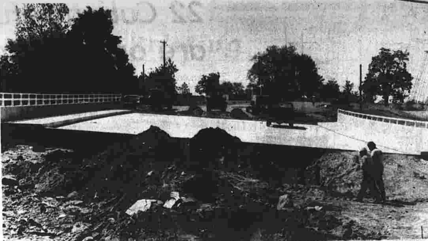
Work progresses on a bridge over the Hockanum River at Deming Street and Tolland Turnpike. The work is part of the improvements to Interstate 88, which will increase the expressway's width and, eventually, relocate exit 93 from Tolland Turnpike to Buckland Street.
