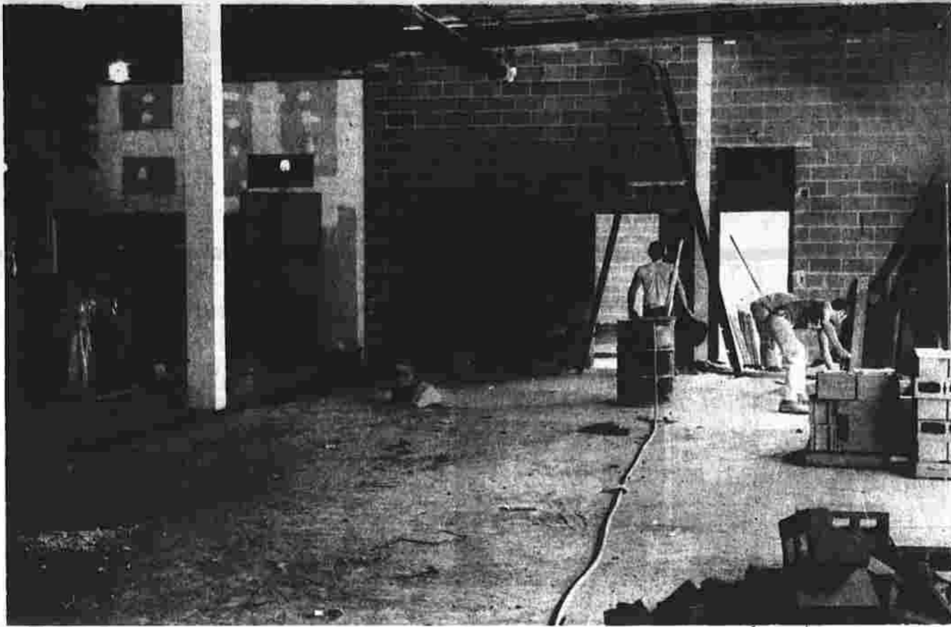
The cafeteria at Howell Cheney Regional Vocational Technical School is being expanded. The brick wall on the right is the new part of the cafeteria, and the white wall on the left is the old cafeteria. (Herald photo by Pinto)
